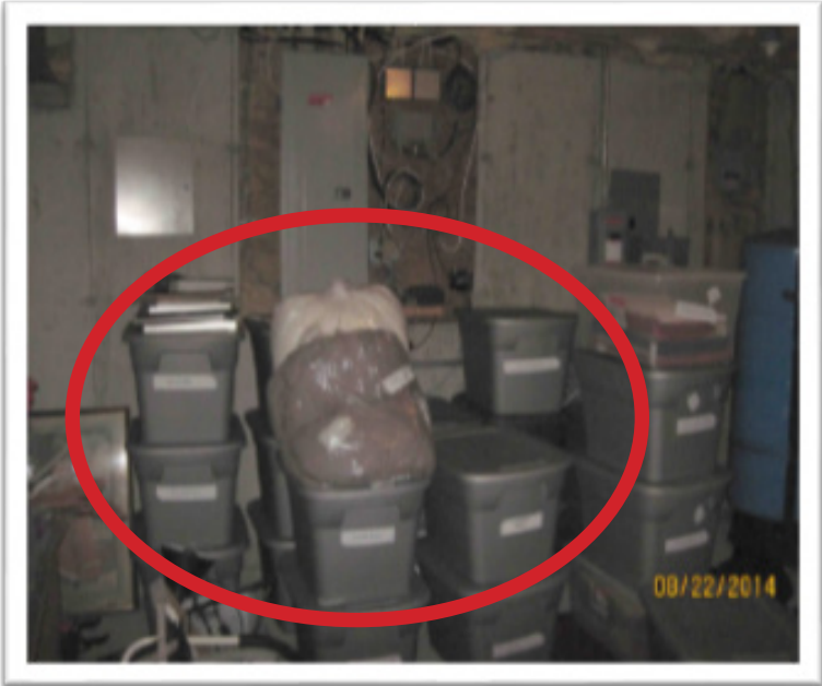
Photo D3: Working clearance not maintained: NEC 110.26
